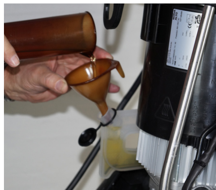
Pump oil tank with oil level sight and fill/empty function.
